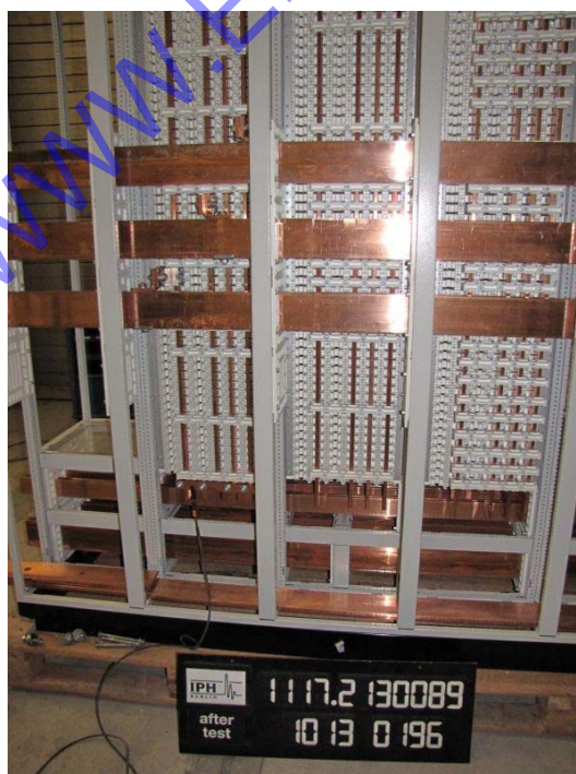
Photo 8: Test object after the verification of short-circuit withstand strength of busbar F4 in panel 2
