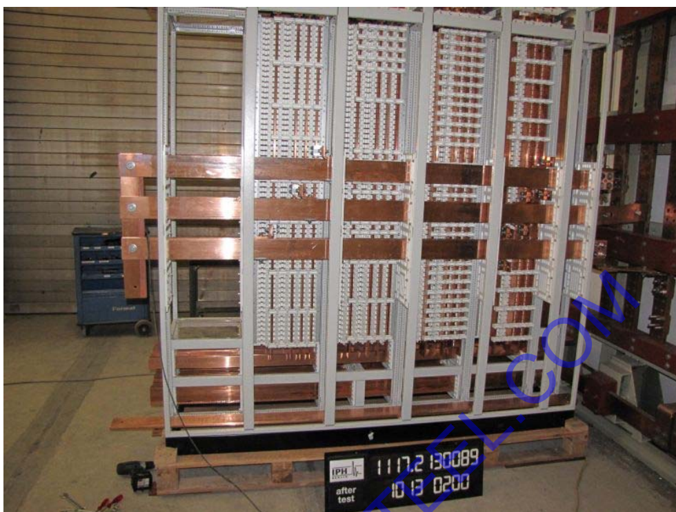
Photo 9: Test object after the verification of short-circuit withstand strength of busbar D in panel 2
