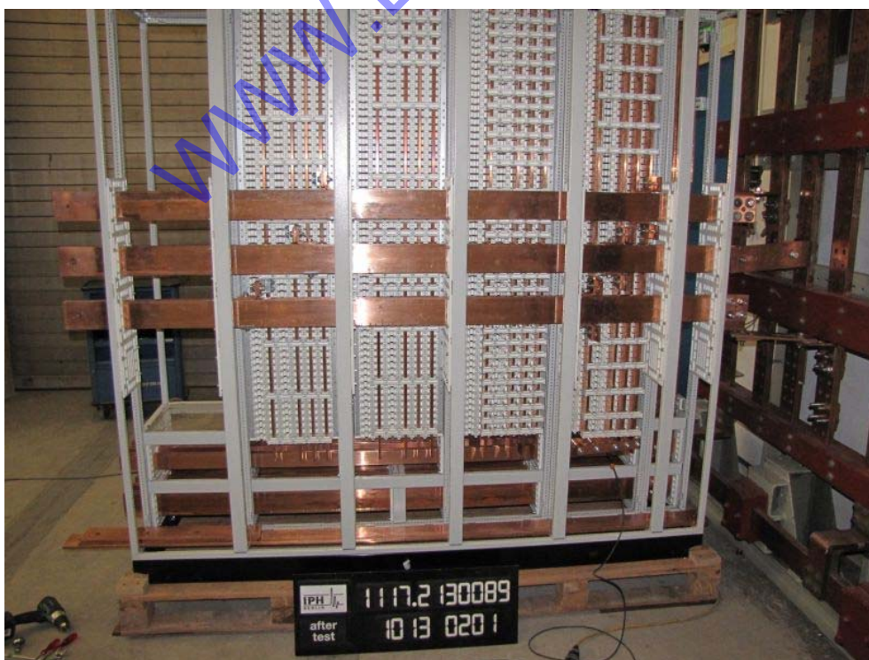
Photo 10: Test object after the verification of short-circuit withstand strength of busbar F1 in panel 2
