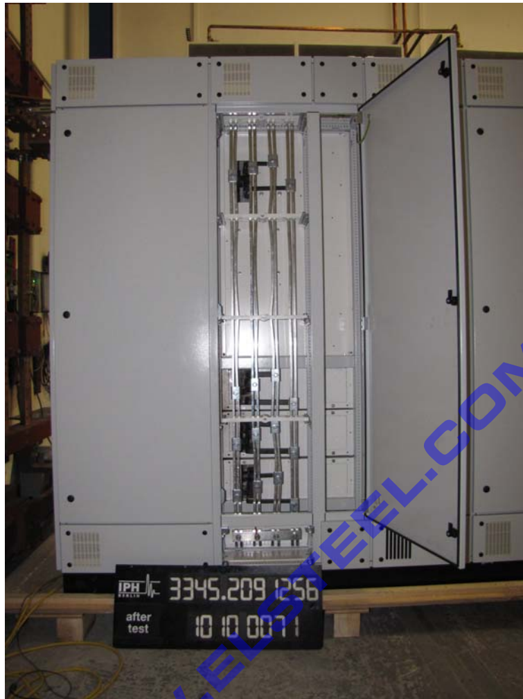
Photograph 8: Test object after test of short-circuit withstand strength of the neutral of the distribution busbar
