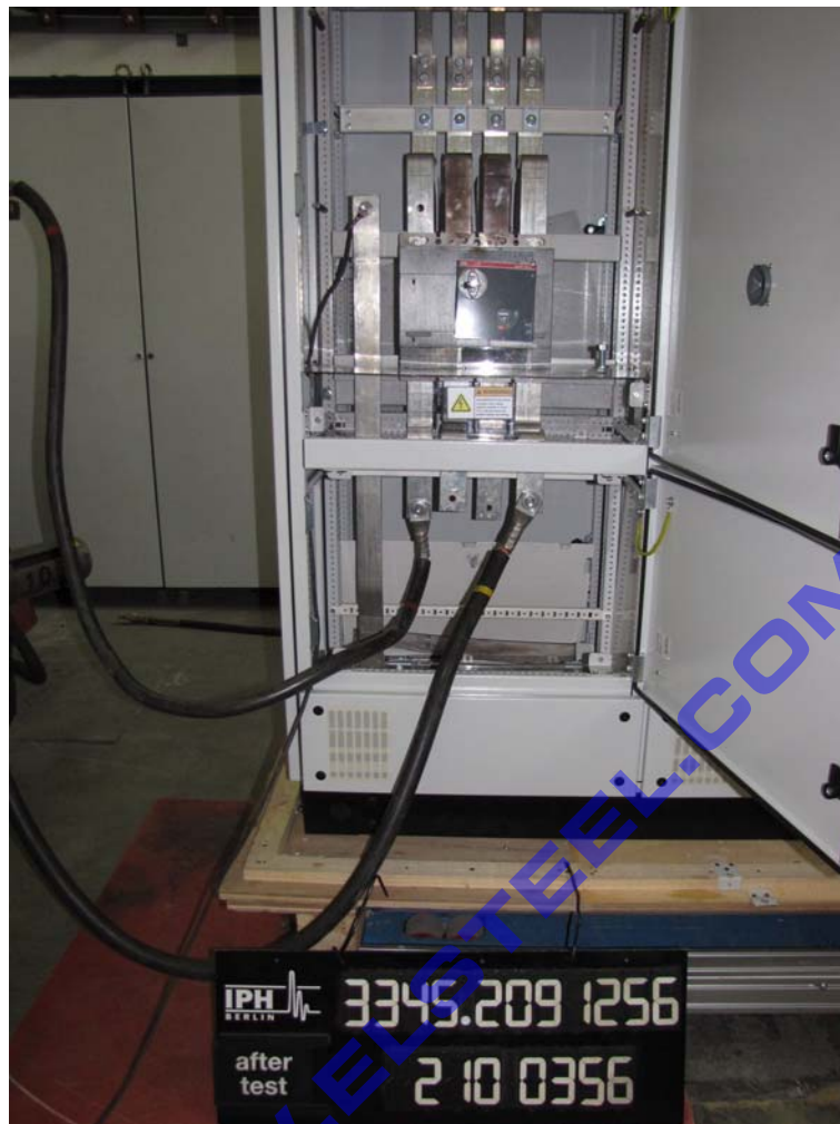
Photograph 10: Connection to the test object for test of the neutral of outgoing MCCB-feeder
