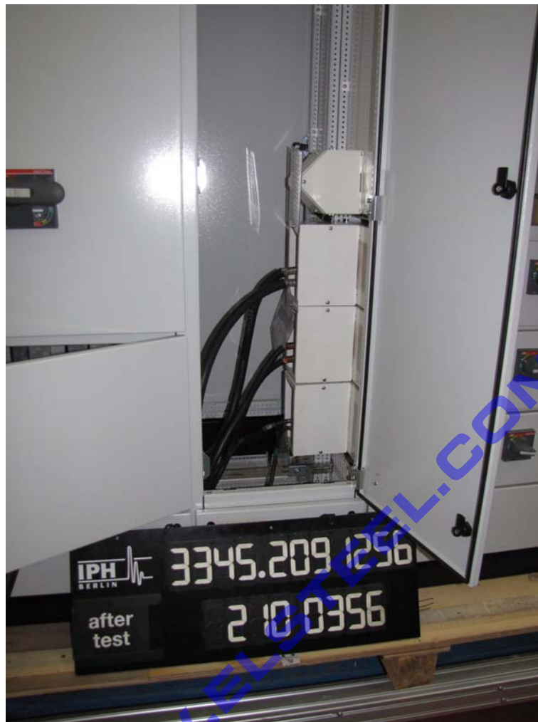
Photograph 11: Short-circuit connections for test of the neutral of outgoing MCCB-feeder
