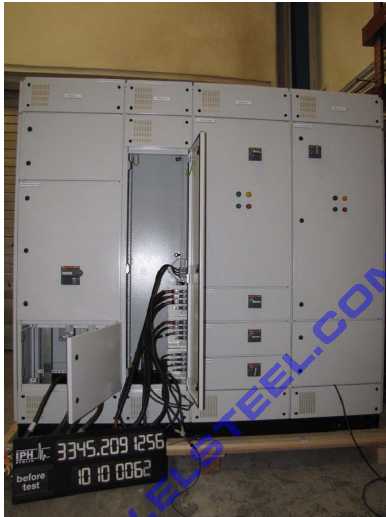
Photograph 4: Connection of the MCCB-feeder for the verification of the conditional short-circuit current
