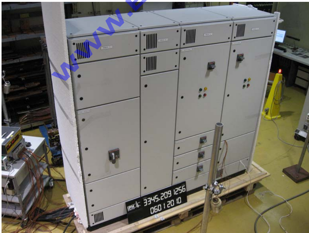
Photograph 2: Front view of test object in the temperature-rise test room
