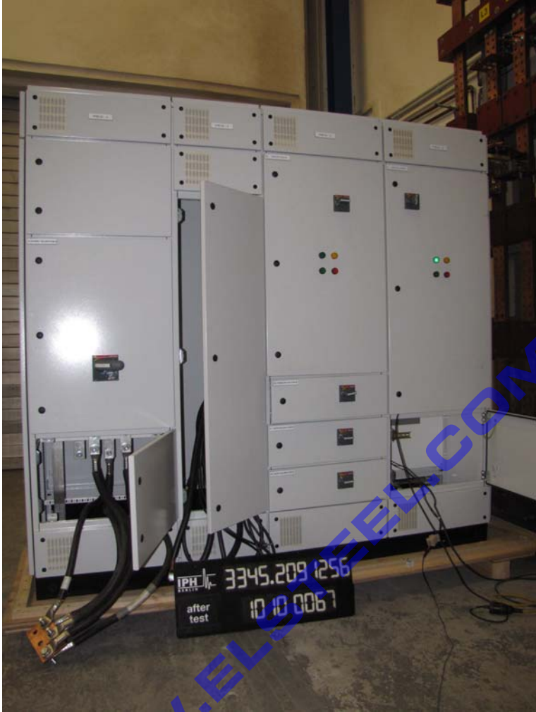
Photograph 5: Test object after short-circuit test 1010 0067
