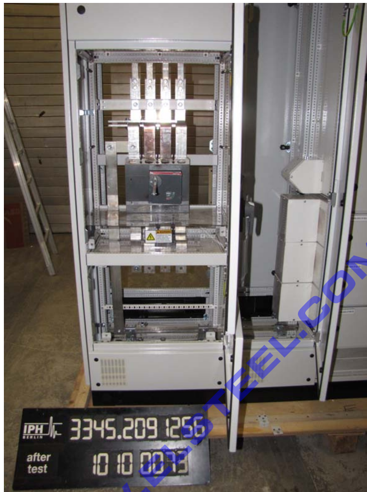
Photograph 9: Test object after test of short-circuit withstand strength of the PE busbar
