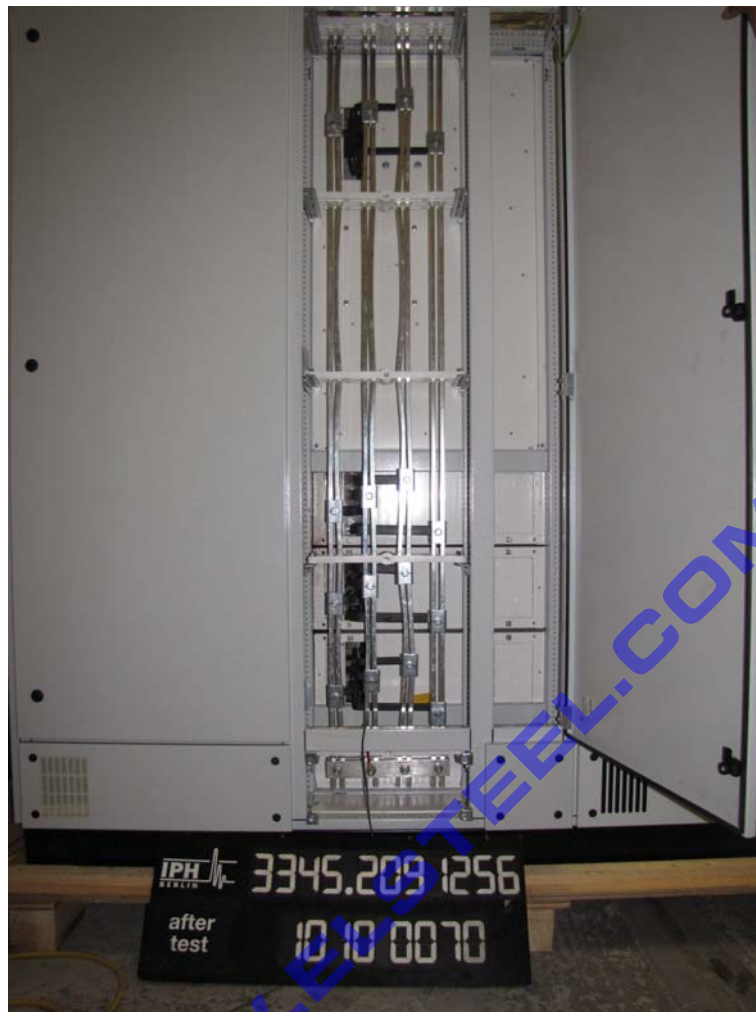
Photograph 7: Test object after test of short-circuit withstand strength of the distribution busbar
