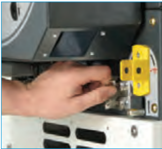
4 Lock the earthing switch by the key (if available)
