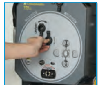
12 Close (ON) the vacuum circuit breaker
