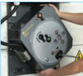
7 Close the air rotary isolator by the rotation
