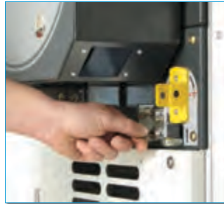
2 Unlock the earthing switch by the key (if available)
