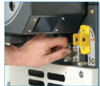
8 Unlock the earthing switch by the key (if available)
