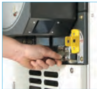
10 Lock the earthing switch by the key (if available)
