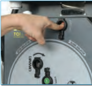
1 Open (OFF) the vacuum circuit-breaker
