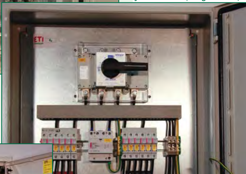
DC junction box (CH gPV fuses)
