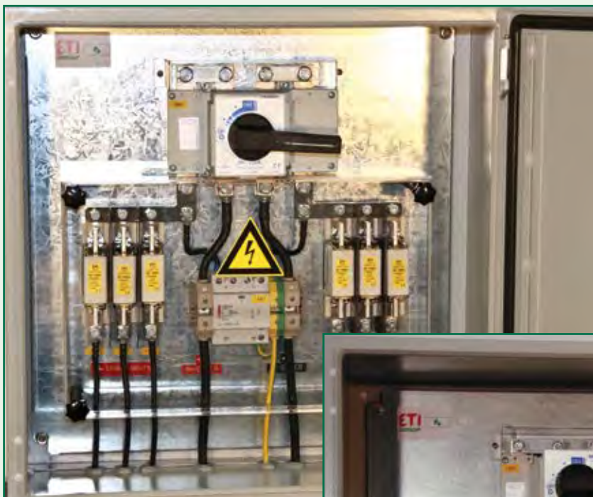
DC junction box (NH gPV fuses)
