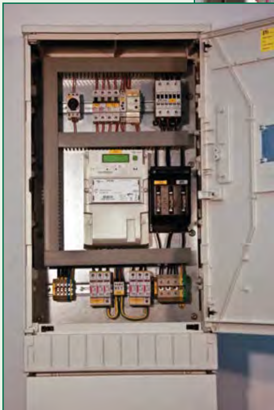
Meter distribution cabinet
