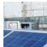
ITALY Cooling loop flow & temperature control
