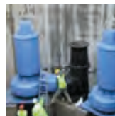
IRELAND Maintaining pressure at pumping stations
