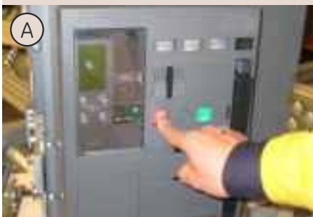
Fig. A: Press the off button on the breaker Fig. B: Key lock key rotate anti clock wise Fig. C: Device locked out
